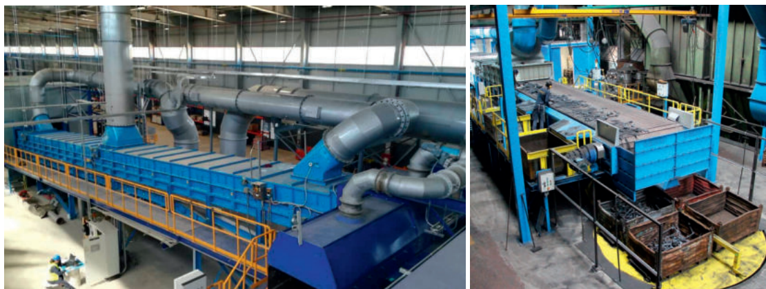
MCCs installed in two different foundries: MTI in Mexico (left) and Pilenga Baldassarre in Italy (right).
