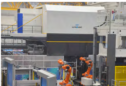
The extraction hood captures the smoke and aerosol mist directly above the die casting machine. The energy-efficient treatment of the exhaust air then takes place via the Ultravent electrostatic precipitator (to the left of the hood).
