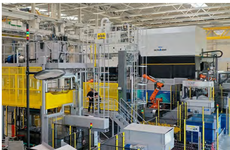
The 4,400-tonne casting cell with energy-efficient KMA exhaust air technology in newly built DGS pattern foundry in St. Gallen, Switzerland.
