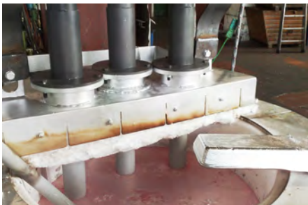
Immersion heater in holding furnace.
